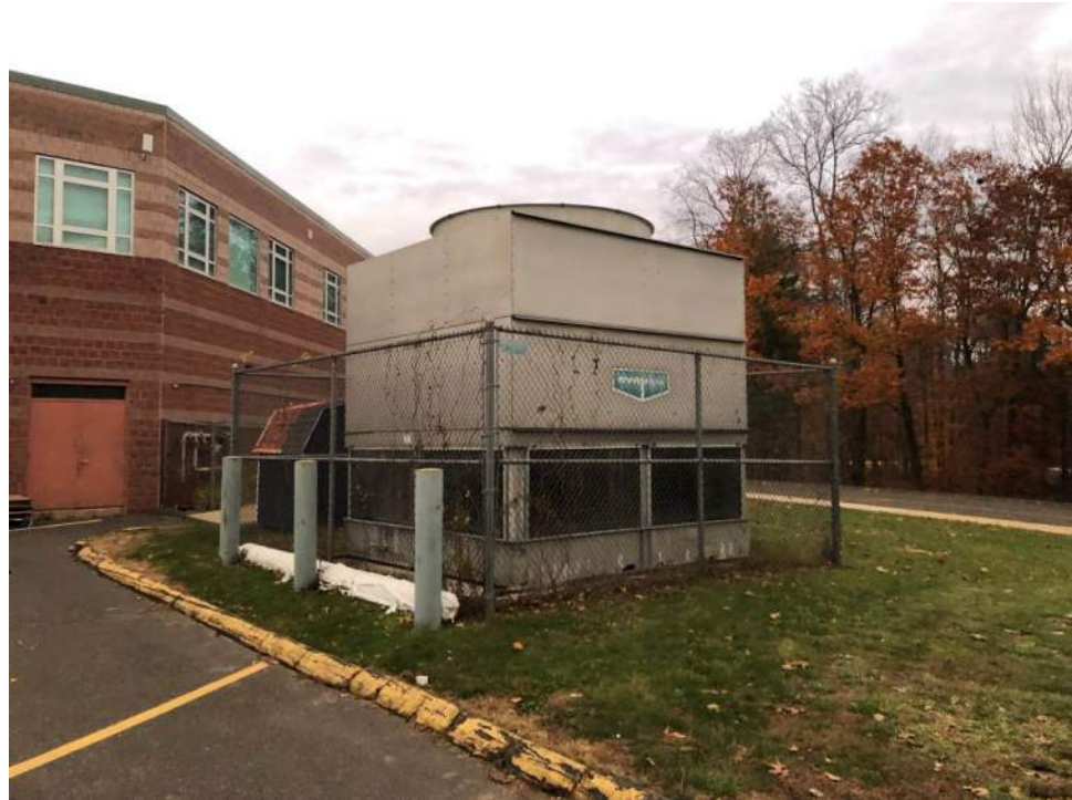
Existing Evapco cooling tower at or past its useful life.
