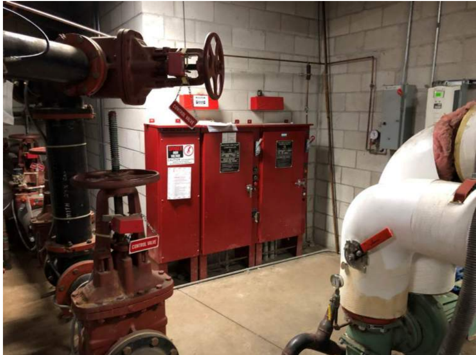
Obsolete fire pump controller.
