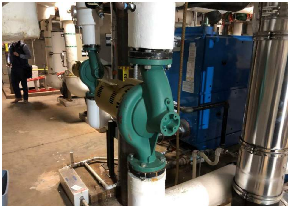
Boiler primary pumps in good condition.
