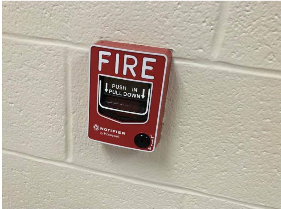
Newer fire alarm pull station.
