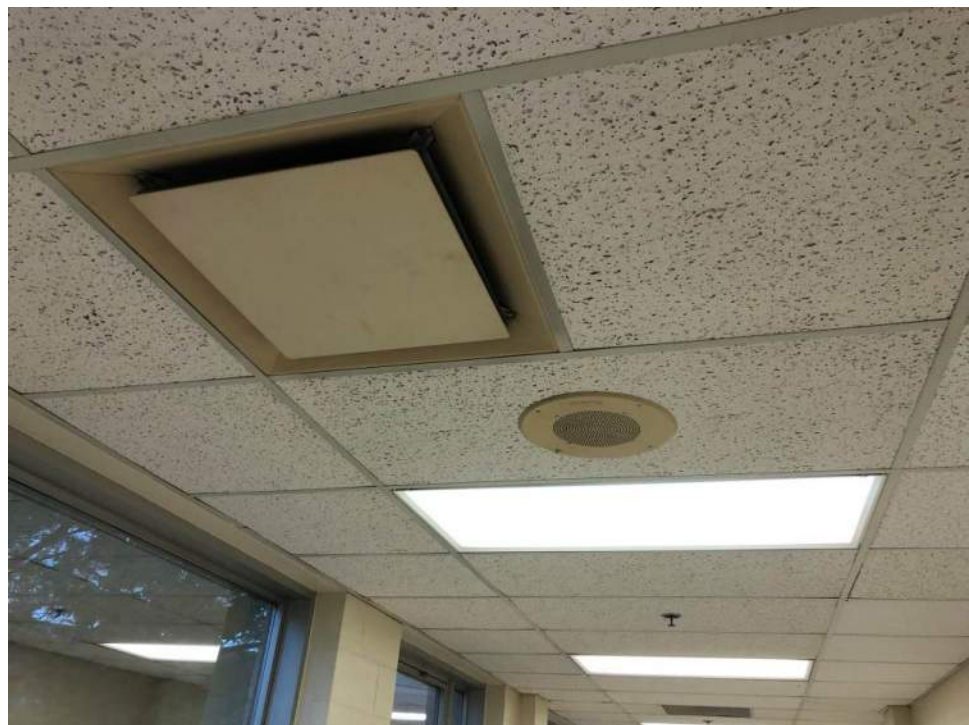
Example of dated-looking supply diffuser.
