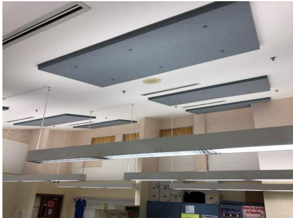
Example of classroom pendent fluorescent lighting.
