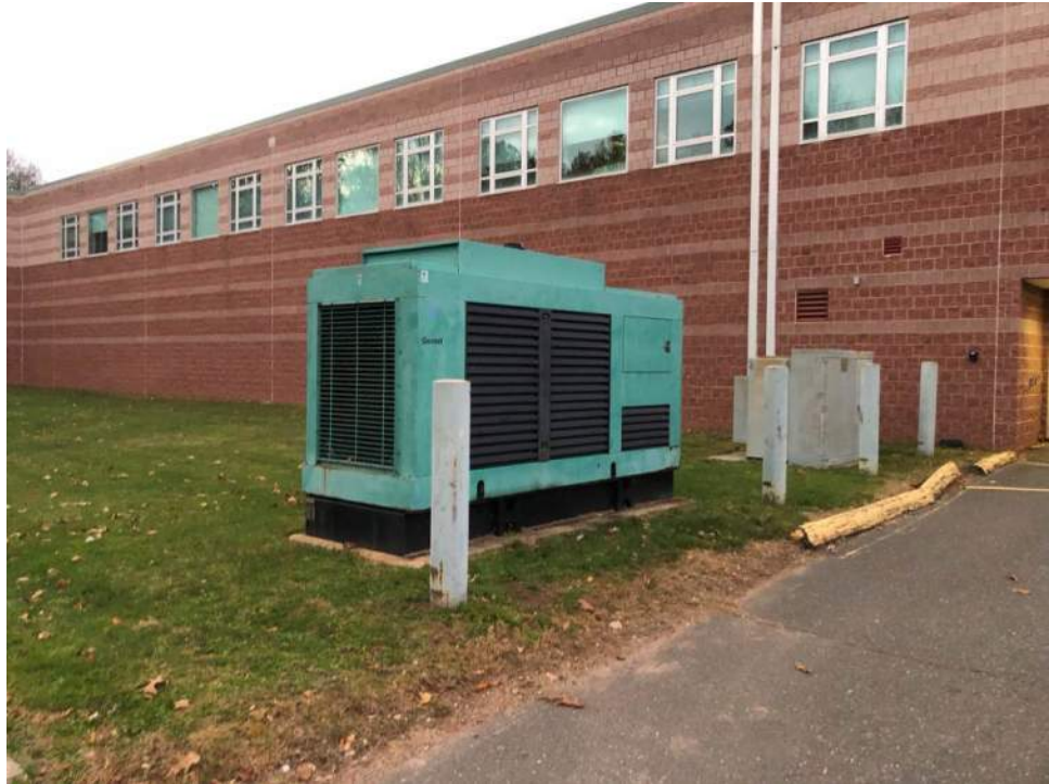
Diesel generator with belly tank.
