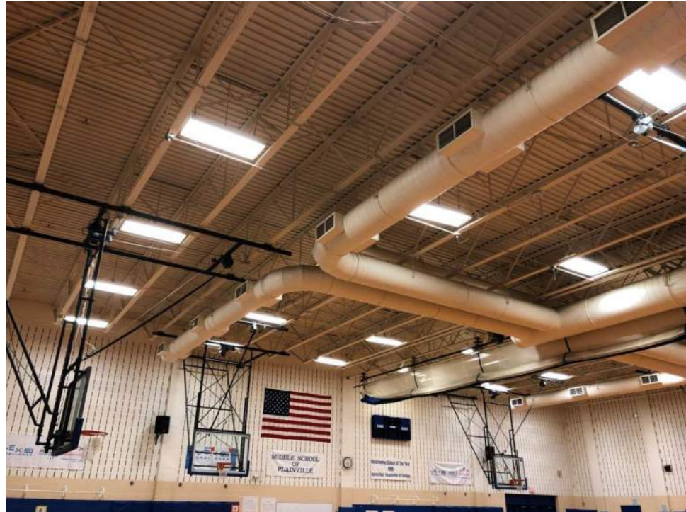
High bay gym lighting.
