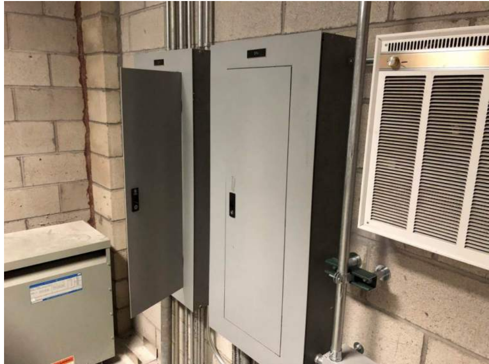
Existing electrical distribution panelboards.
