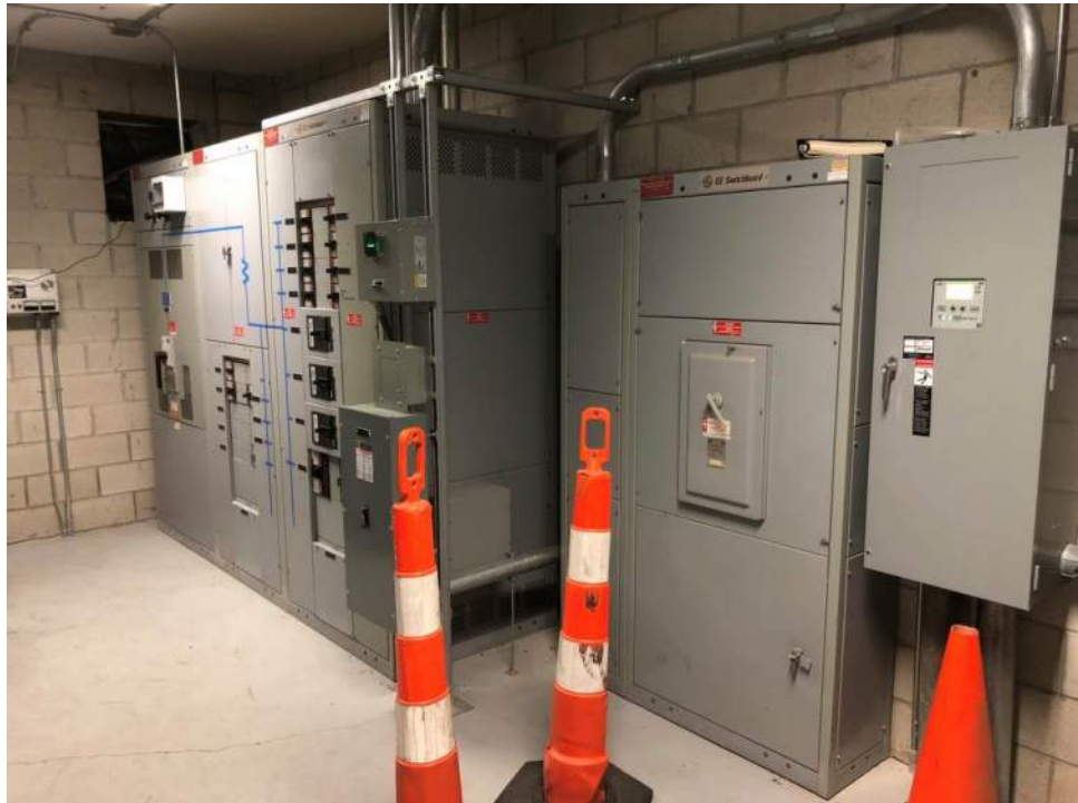
Main switchgear, original to building and near the end of its useful life.
