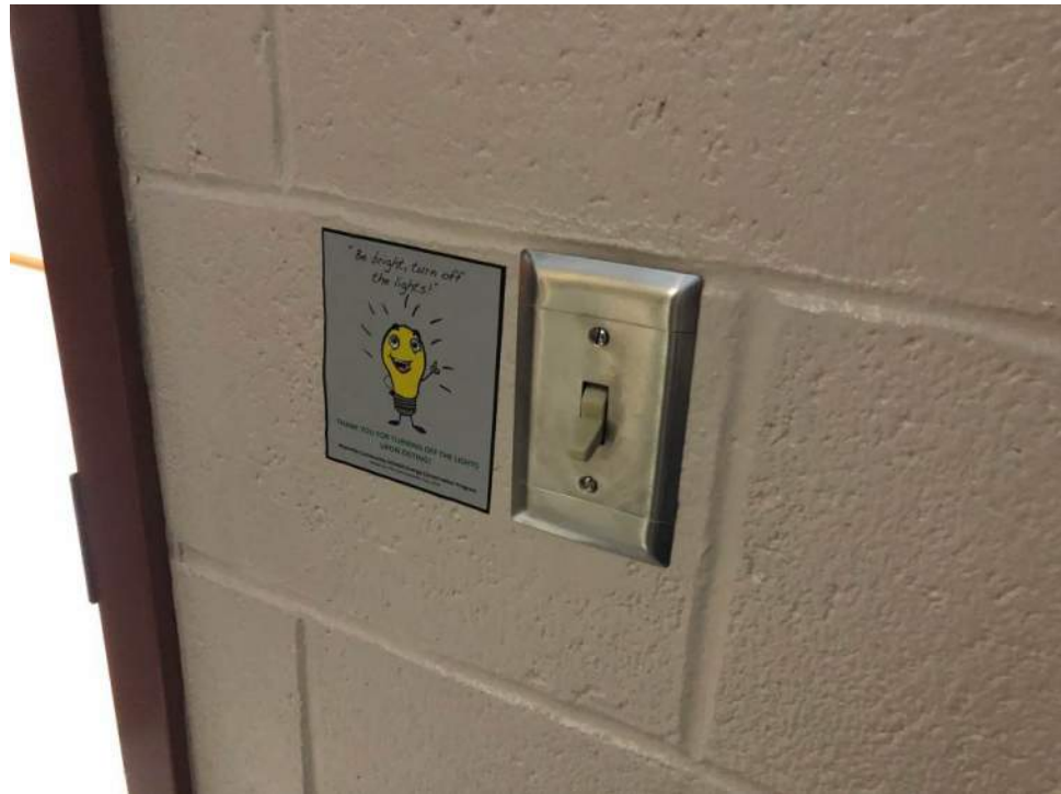
Example of manual toggle switch for lighting control.
