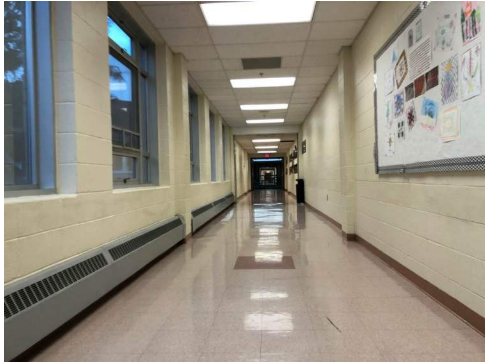
Example of corridor 2 x 4 fluorescent lighting.
