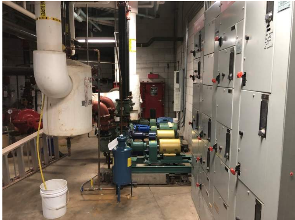
Heating hot water secondary pumps in fair condition.
