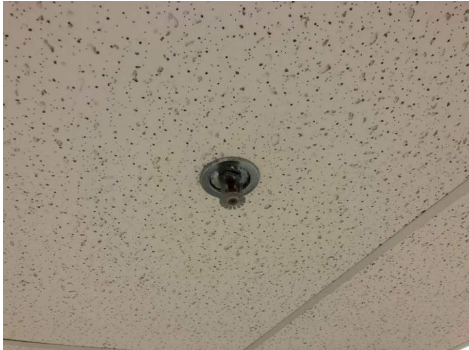
Example of pendent sprinkler head.
