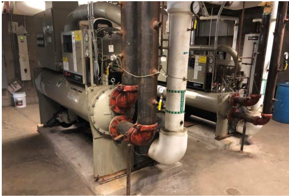
Existing 300-ton and 150-ton Trane screw chillers, at or past their useful life.
