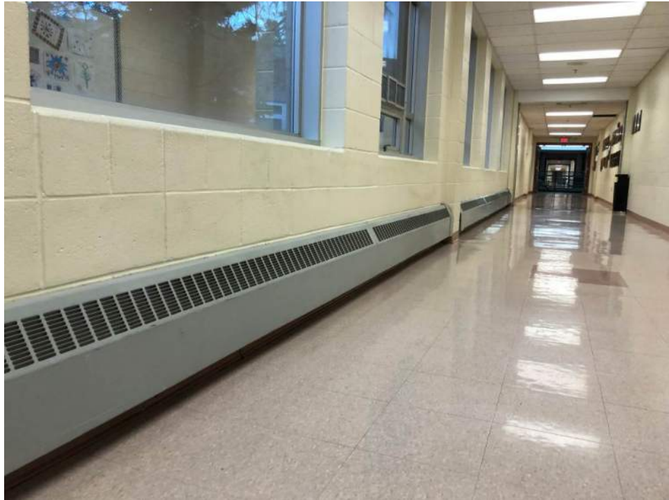
Example of perimeter fin-tube radiation in a corridor in fair to good condition.
