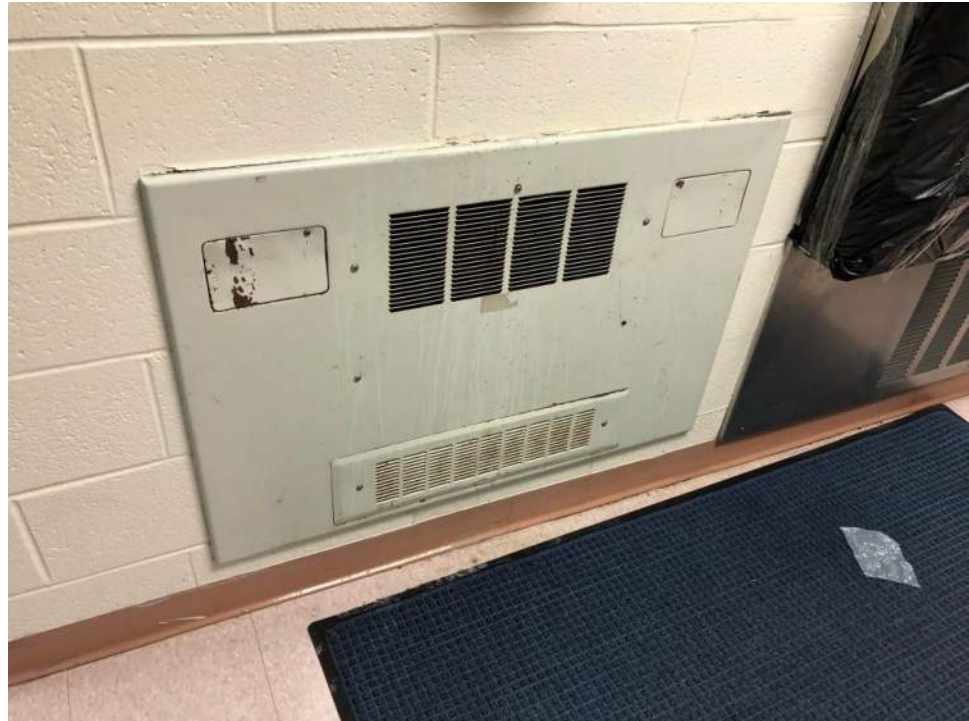
Example of cabinet unit heater in fair condition, showing wear and tear.
