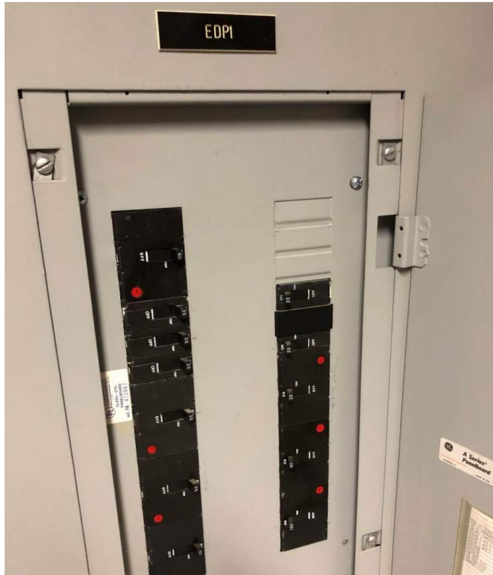
Circuit breakers Inside an existing electrical distribution panelboard.
