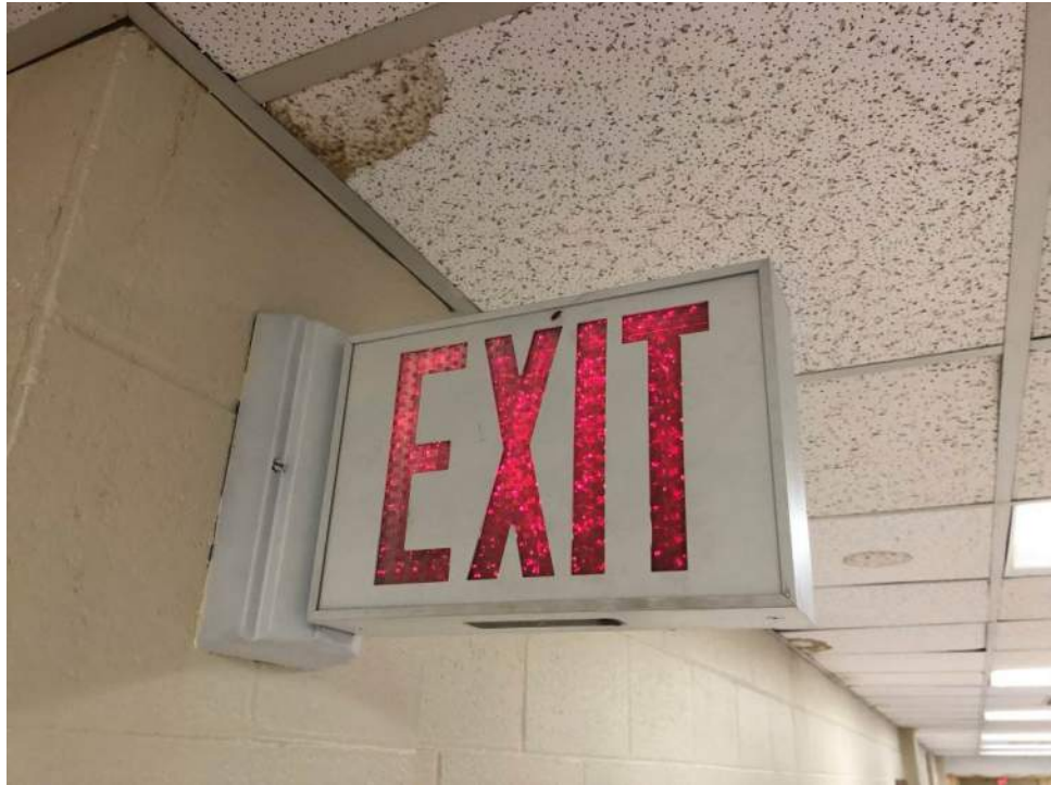
Example of existing exit sign.
