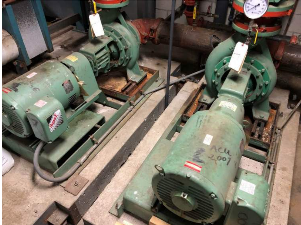
Existing condenser water pumps, at or past their useful life.
