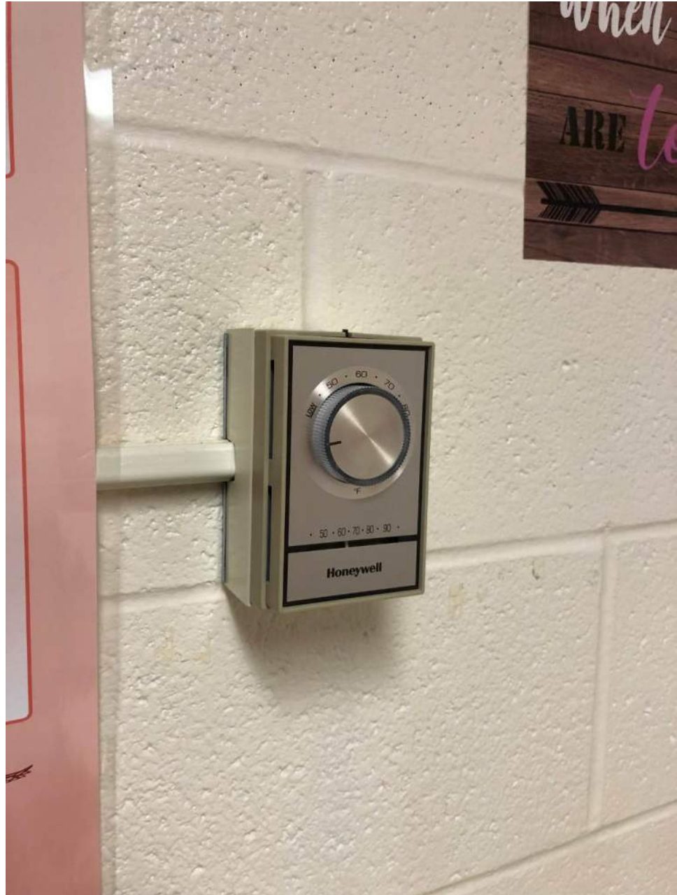
Example of existing outdated thermostat.
