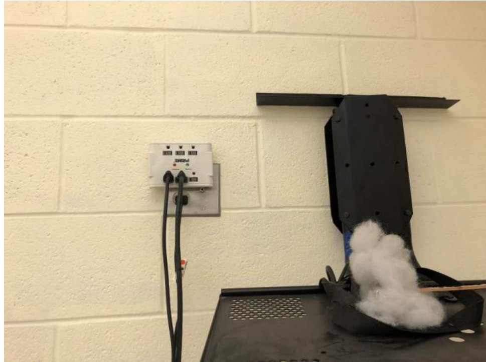
Example of existing power receptacle.
