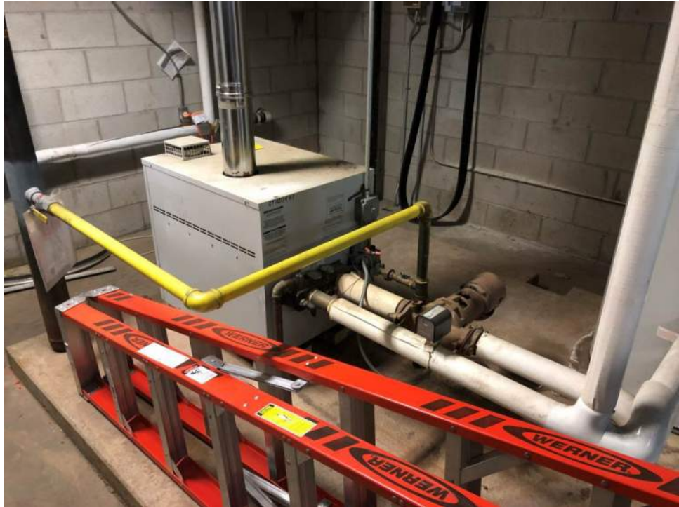
Lochinvar semi-instantaneous hot water heater.
