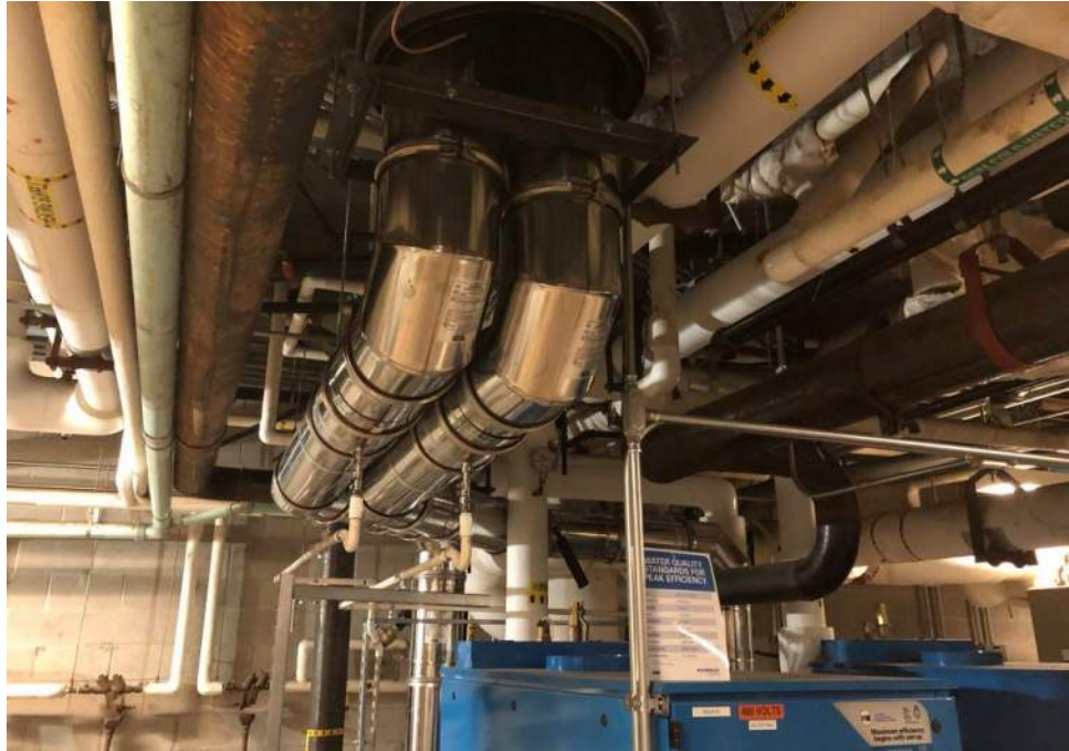
Stainless steel double wall independent boiler flues going up to the roof inside the existing boiler breaching.
