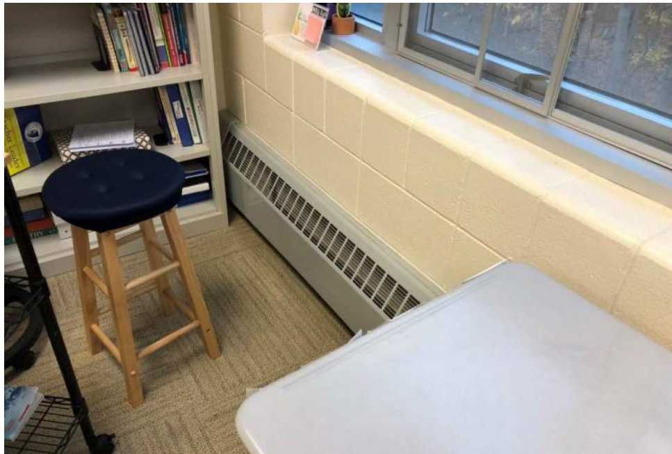
Example of perimeter fin-tube radiation in a classroom in fair to good condition.
