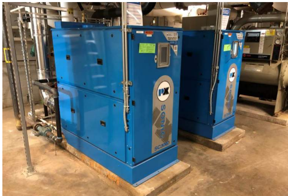
Recently installed Patterson-Kelley gas-fired condensing boilers in excellent operating condition.
