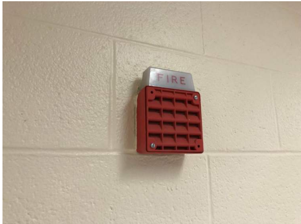
Older fire alarm horn/strobe.
