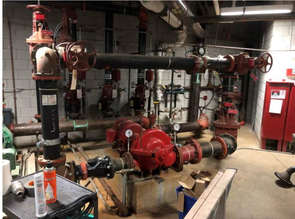
Fire service piping and horizontal electric fire pump.
